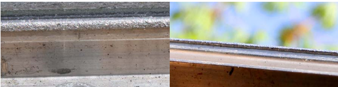
Beech Hurst rail soon after installation - Top view (picture above left) and the view looking up (picture above right) at the edge of the rail, note the large amount of edge burr.
