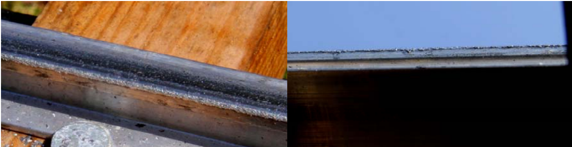
Commercial rail soon after installation - Top view (picture above left) and the view looking up (picture above right) at the edge of the rail, note the small amount of edge burr.
